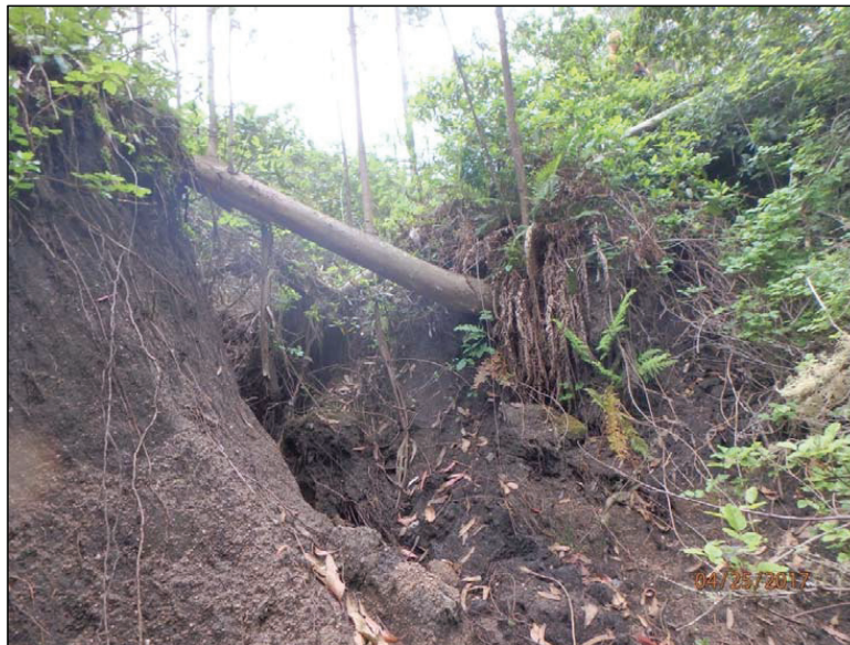
Photo 18 (Site #40): View of active hillslope gully below Site #40 looking upstream. This photo was taken from the edge of the tree-line near the headwaters of a small Class III stream that drains to Site #16 downstream. The gully is conveying sediment from the gully erosion upslope to the Class III stream.
