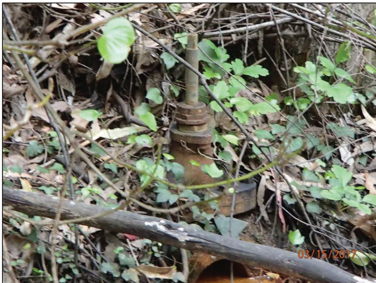
Photo 8 (Site #4): View of the seeping drainage valve at base of the dam fillslope in the axis of the valley downstream of pond.
