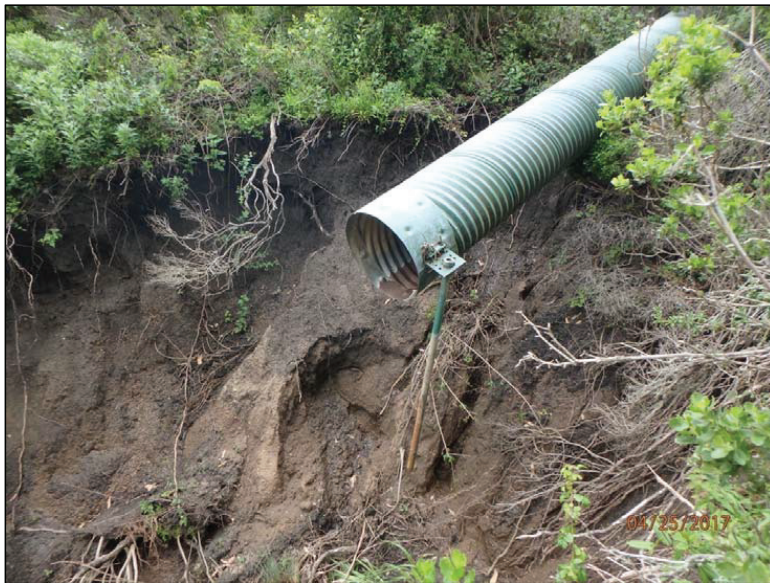
Photo 16 (Site #40): View of a section of disconnected culvert downspout at the top of an actively migrating headcut and gully below the paved Private Drive at Site #40. Oxidation exposed on the stake is indicative of the previous depth of burial prior to the episodic hillslope failure.
