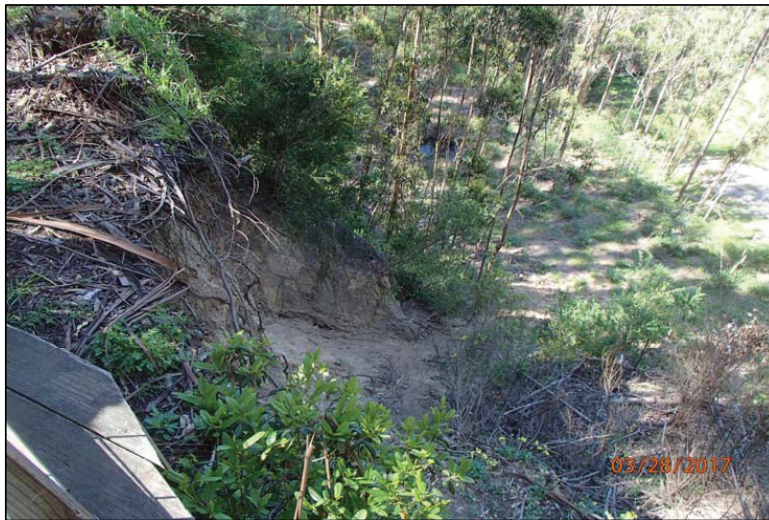
Photo 34 (Lookout Vista): View of the failing hillslope below the wooden lookout vista platform. The quarry cutslope is oversteep and is actively failing in multiple locations along the upper edge of the quarry area.
