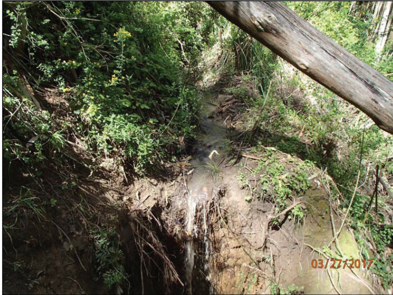
Photo 7 (Site #4): View of a road fill failure caused by diverted pond outflow. This erosion feature is located down the right road from the levee. Note the road prism is completely washed out.
