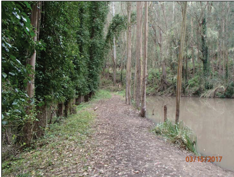
Photo 5 (Site #4): View of the levee associated with the on-stream reservoir Site #4, looking west-southwest across the top of the dam face.
