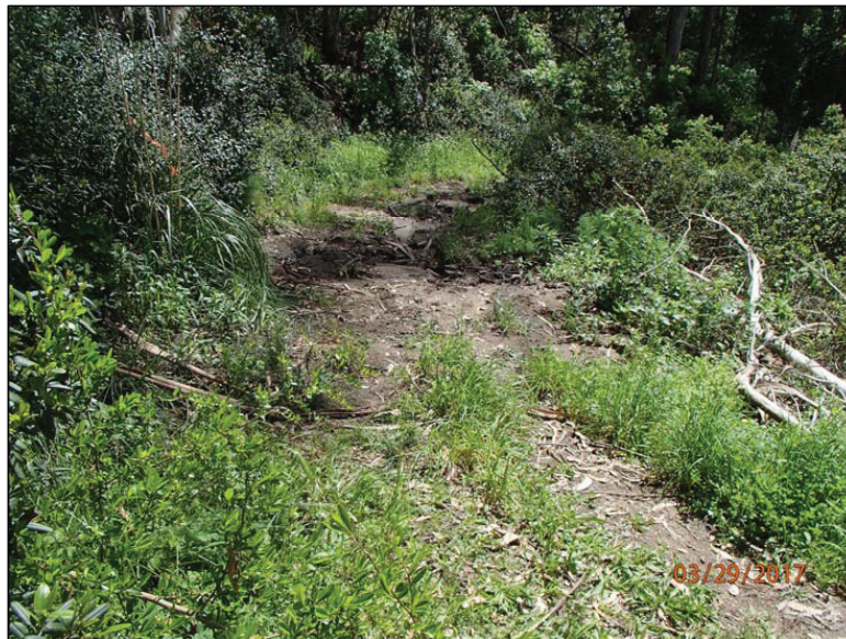
Photo 22 (Site #16): View of the fill crossing at Site #16 on the Dolphine Fire Road. Diverted stream flow is actively eroding gullies down the left road from this stream crossing.
