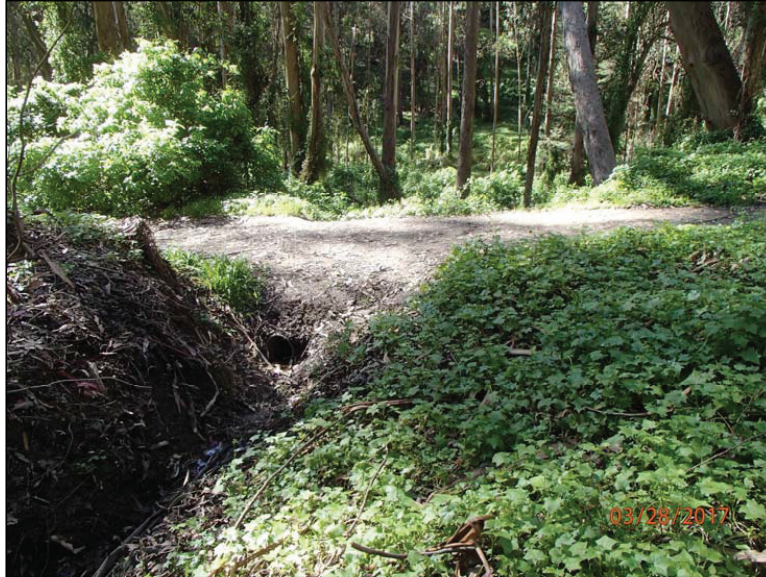
Photo 27 (Site #36): View of a culvert inlet on a small Class III stream at Site #36. This site is downstream of the pond Site #37 in the base of the quarry.
