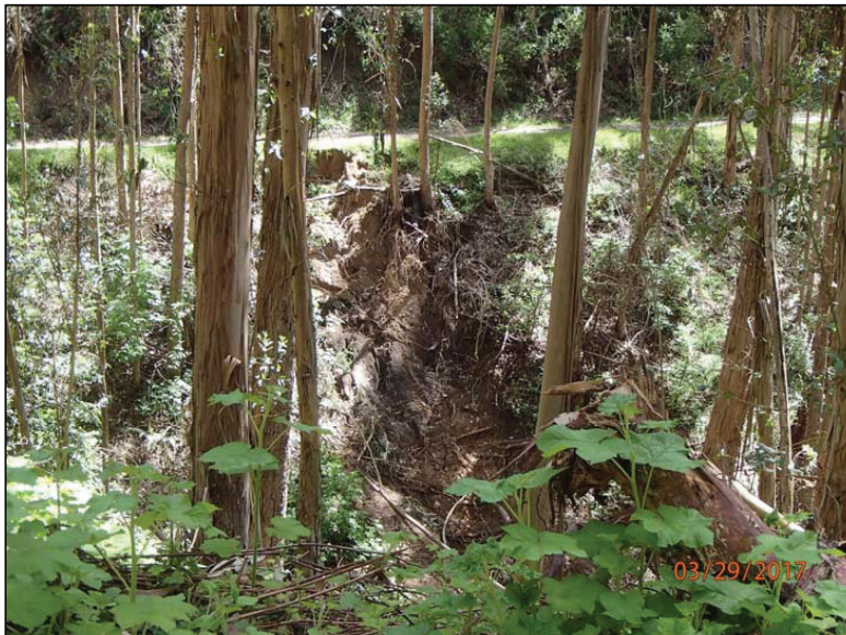
Photo 14 (Site #39): View of an outboard fill failure to the left of the stream crossing. The fill failure was induced by the diverted streamflow from the plugged stream crossing at Site #39 and excessive concentrated road surface runoff.
