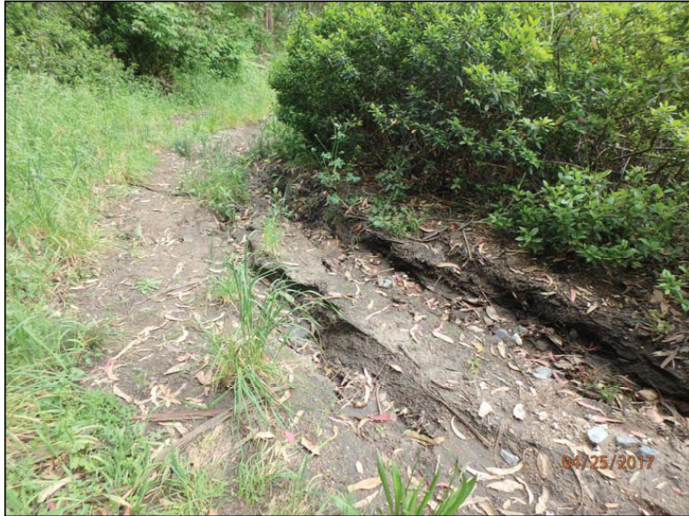
Photo 23 (Site #16): View of the left road approach to fill crossing Site #16. Diverted stream flow is actively eroding gullies down the left road from this stream crossing and delivering to a watercourse at Site #15.
