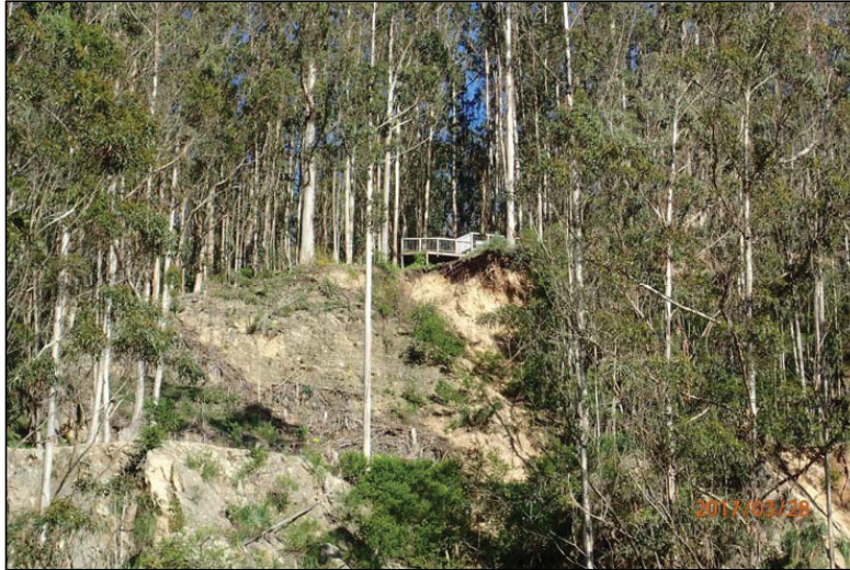
Photo 33 (Lookout Vista): View of the lookout deck and failing hillslope below the outermost footing. This photo was taken looking upslope from the base of the quarry floor.
