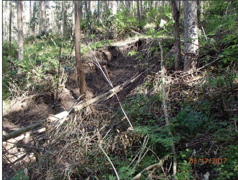
Photo 11 (Site #19): View of failing cutbank immediately upslope of the right edge of stream crossing Site #19. This cutbank failure delivers directly to the Class III stream in the axis of the crossing fill crossing.
