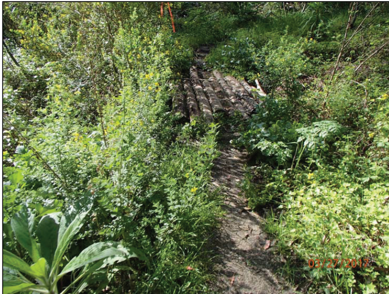
Photo 25 (Site #24): View of a makeshift foot bridge at stream crossing Site #24. The active erosion at this site is minimal, and a formal crossing should be established.
