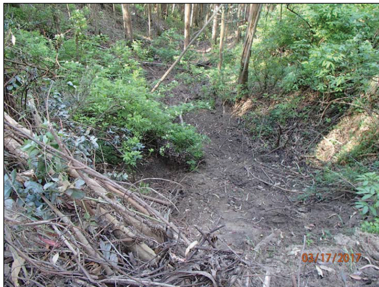
Photo 12 (Site #19): View of failing outboard fillslope, looking downslope at the fill failure deposits below the right hingeline of the fill crossing at Site #19. This photo was taken from the outboard edge of the road.
