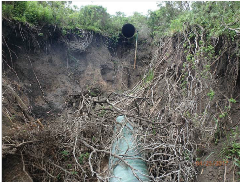
Photo 17 (Site #40): View looking upslope at the same disconnected downspout and active erosion as shown in the previous photo. The photo was taken from the base of the gully downslope of the headcut standing on top of one of the failed sections of culvert.
