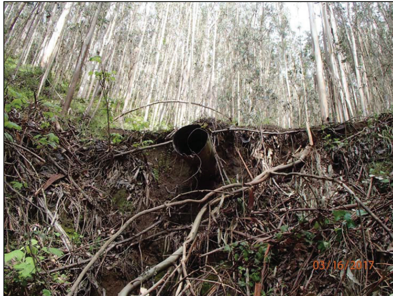
Photo 21 (Site #9): View of the perched culvert outlet at stream crossing Site #9. The culvert at this crossing is undersized and installed high and short in the fill with a 6ft drop at the outlet and subsequent outboard fill erosion.
