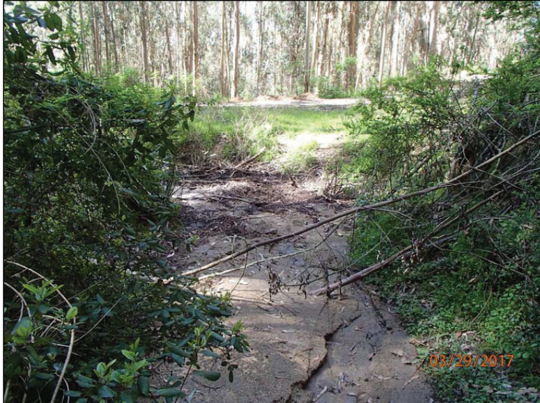
Photo 13 (Site #39): View looking downstream from the upstream extent of the of the failing stream crossing. Note the recently deposited sediments that have plugged the culvert inlets. The sediment is causing the stream flow to divert down the left road which is inducing a delivering fill failure.
