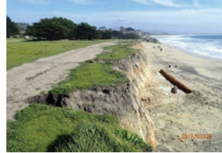
Area of concern example - bluff erosion
