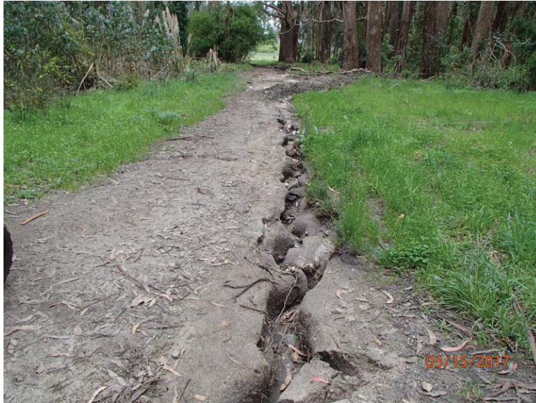
Photo 3 (Meadow Trail): View of active gully erosion along the Meadow trail. Combined diverted stream flow and concentrated road runoff are eroding the road surface along this native surfaced road.
