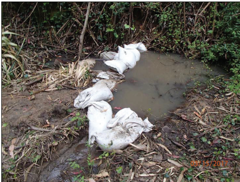
Photo 6 (Site #4): View of temporary dysfunctional sandbag spillway at the southwest corner of the on-stream pond Site #4.
