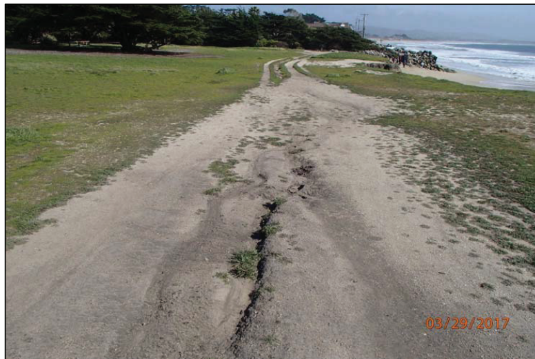
Photo 32 (Coastal Bluff Trail): View of road surface erosion along the coastal trail due to concentrating runoff. Note the exposed beach protection rock armor at the edge of the park boundary in the distance.
