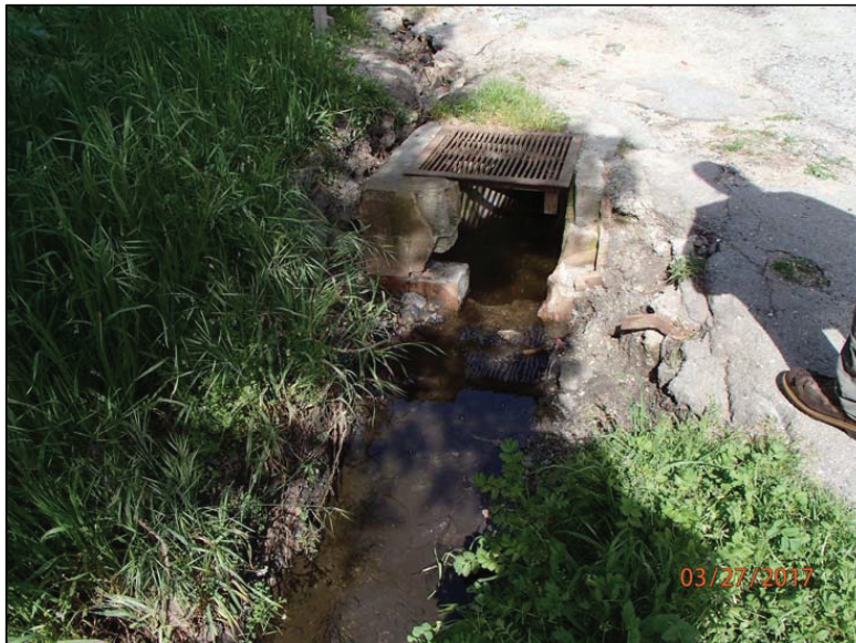
Photo 24 (Site #23): View of the outlet of the culvert at stream crossing Site #23 at the edge of the main parking lot. This culvert is undersized and stream flow avulses out of the drainage alignment and onto the parking lot surface.
