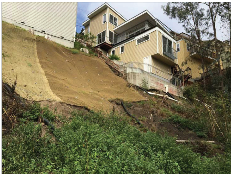
Photo 20 (Site #41): View of a hillslope failure and undermined residences upstream from Site #41. This area upslope extent of AOC 4 as discussed in the text of the report. This photo was taken from the outboard edge of the Fire Break Road upslope from the Upper Pond Legacy Road as shown on Map 2.
