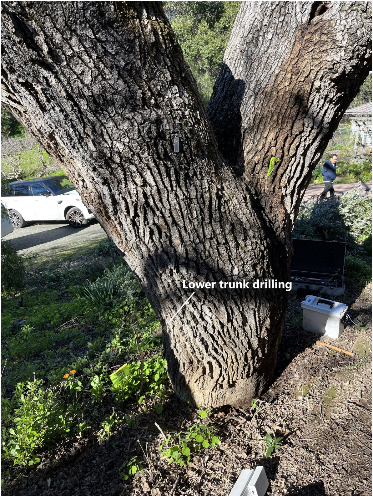
Location of lower trunk resistograph drilling
