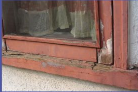
in chipping paint
